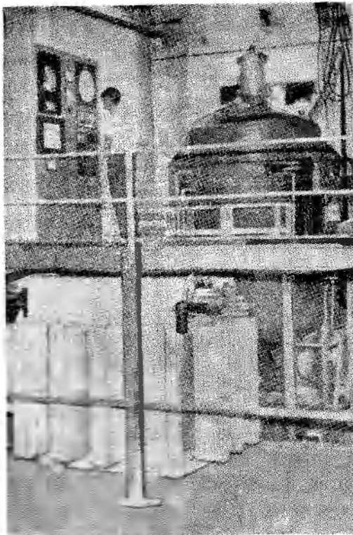
Fig. 2. General view of the Vacuum Furnace, showing the chamber, Transformer and recording panel.
