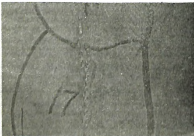
Fig. 6. A weld on the opposite side of this vessel resulted in corrosion in the heat-tinted area
