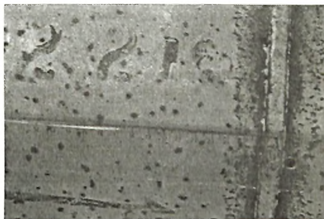
Fig. 2. Iron embedded by a carbon steel wire brush and construction work in the same area has initiated pitting corrosion on stainless steel pipe.
