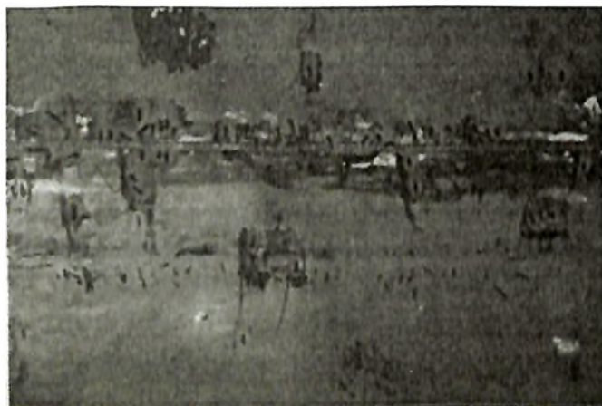
Fig. 4. Weld spatter resulted in corrosion; weld repairs were required after the affected spots were ground out
