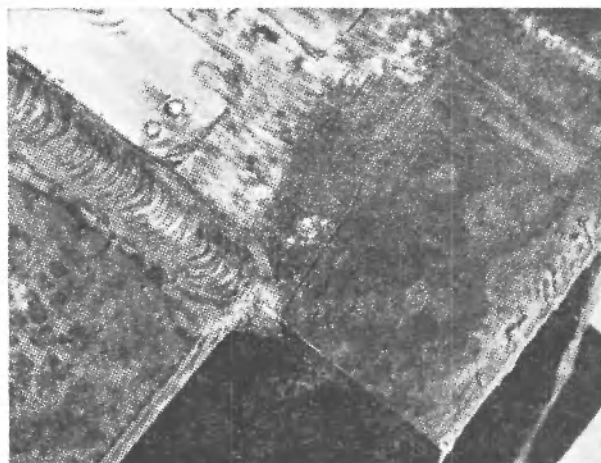
Failure at weld end.
