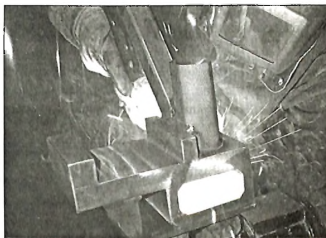
Fig 1. The author MIG welding a thick 6xxx series (Al/Mg/Si) extrusion using a 5356 (5%Mg) filler alloy and high current spray transfer settings.
