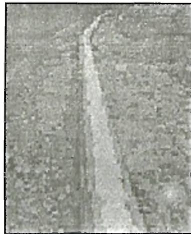
A 320-meter long stainless steel water main pipeline at Mettur, Tamil Nadu. On the right we can see a part of the original main in cast iron. Compare the size.
