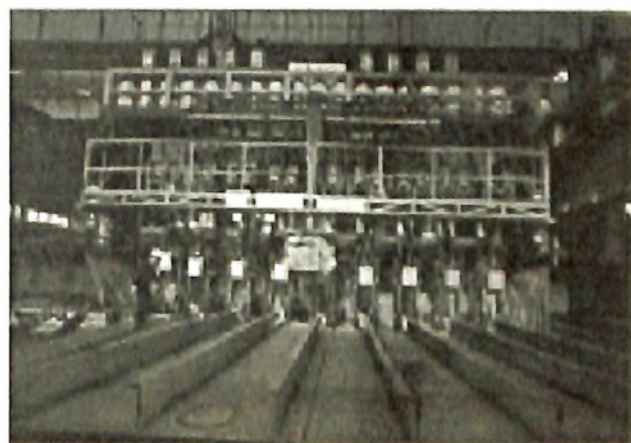
Fig 7. Mechanised cored wire welding system at a shipyard (left – gantry type single torch, right – TAMA type twin tandem with 24 torches)
