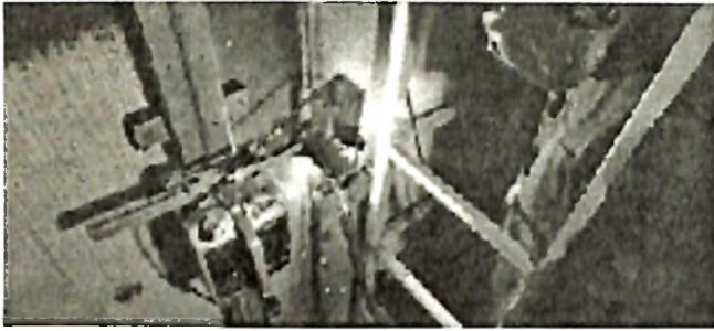
Fig 18. Joint Geometry & Penetration (Top), bead shape(middle) and welding setup (bottom) of V-up welding of 12m thick Chemical Tanker of Duplex SS with 14.27
