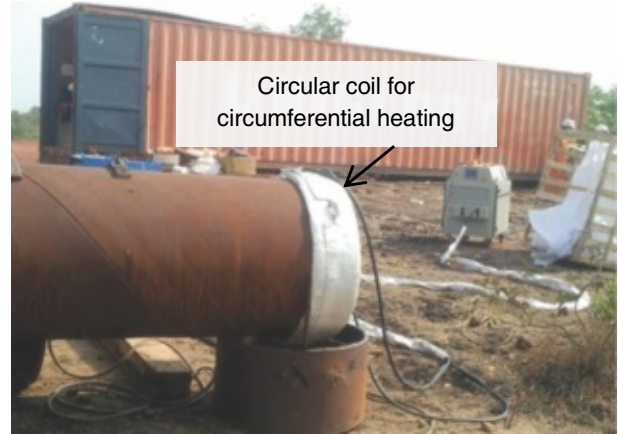
Fig. 2 : Arrangement of induction heater for pre-heating of circular welding joint of pipe
