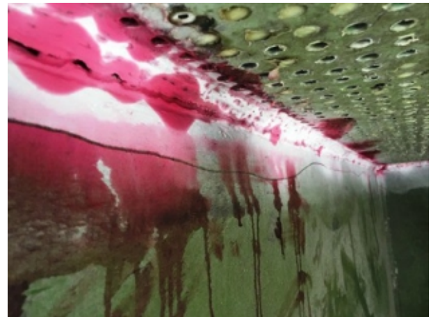
Fig. 1 : Longitudinal Crack on Stiffener Fillet Weld of Sieve Plate can be seen.
