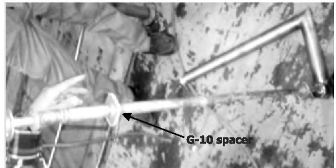
Fig. 6 : Assembly of LN 2 transfer Cryo line
