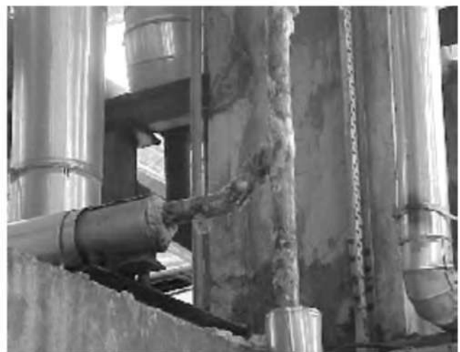
Fig. 4 : Photograph of Hot & cold condensate mixing Tee point after insulation removal
