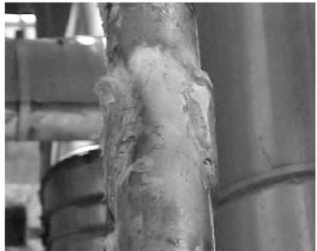
Fig. 3 : Photograph of Leaking portion of the mixing 'Y' joint at RF pad weld joint in 2008
