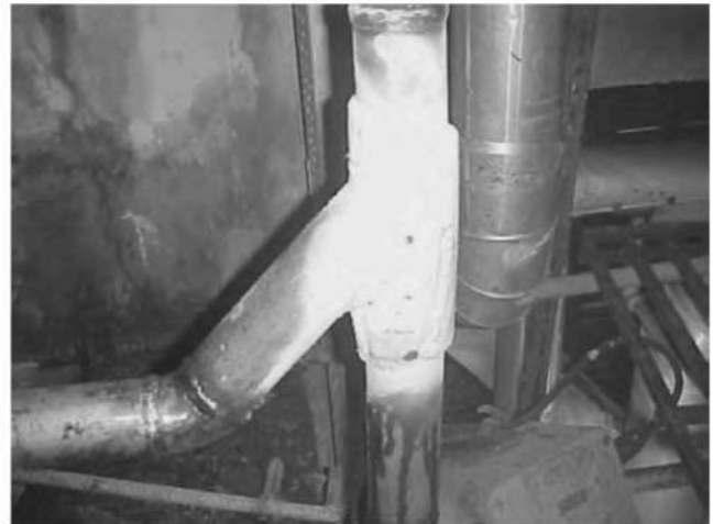
Fig. 2 : Photograph of Replaced mixing point modified to 'Y' joint, DP tested after replacement in 2006
