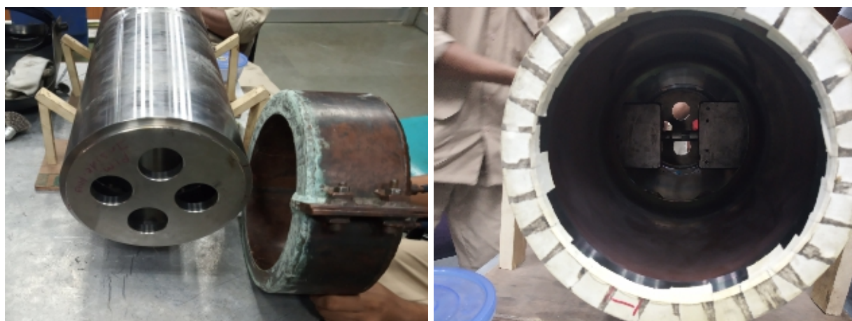
Fig. 4 : Photographs of repair welding done in dissimilar (MDN250 to SAE4130) material motor casings
