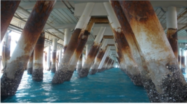
Fig. 4 : Splash Zone Corrosion [38]
