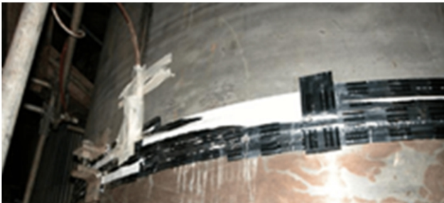
Fig. 3 : A typical purging arrangement of gas flow, conduits affixed by adhesive tape to SS-duplex digester
