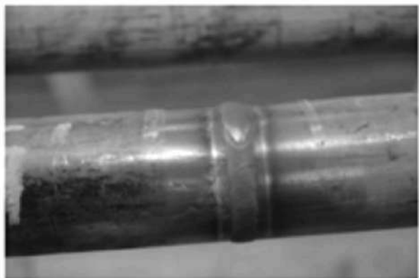
Fig. 11 : A typical boiler tube butt weld made by Orbital TIG
