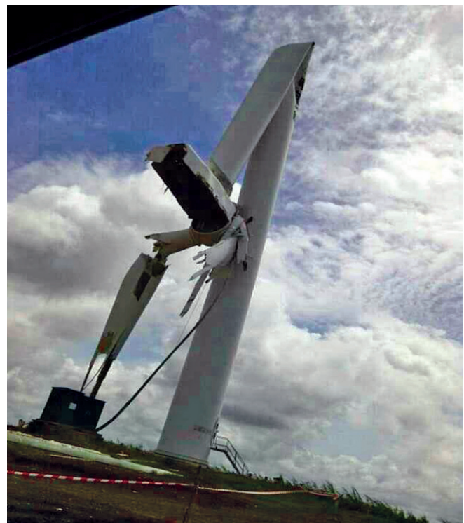
Fig.1 Collapsed tower tube of wind generator caused by typhoon 'catfish'
