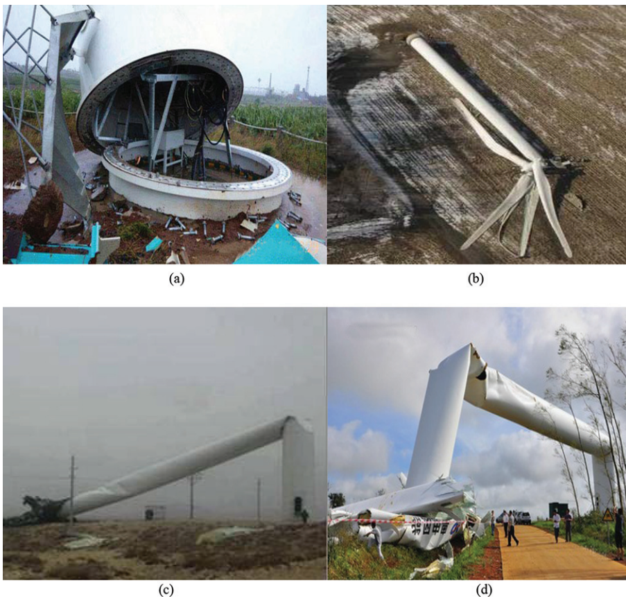
Fig.2 Destruction of tower tube structure of wind generator
