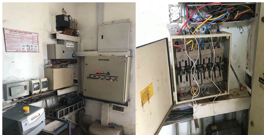
Fig.1: Pictorial view of the efergy with three magnetic probe connected to the central load lines of the transfer switch in the admin block
