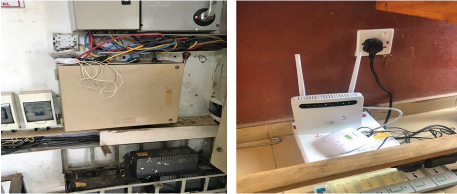
Fig.2: Pictorial view of the efergy transmitter connected to the transfer switch and the efergy router connected to meter in the admin block
