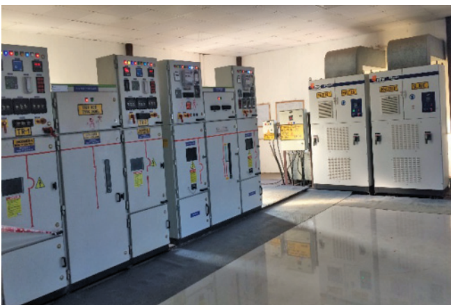
Fig.6: Overall Inverter connection at Dalmia solar power plant
