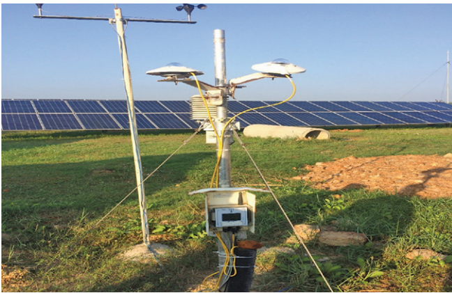
Fig.5: Paranomater used at Dalmia solar power plant
