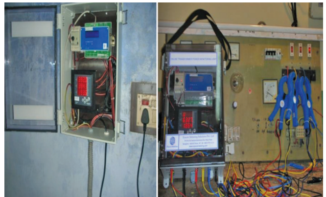
Fig.5: Advanced energy meter connection arrangement at NLCIL-CARD
