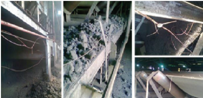
Fig.5: Damage of LHS cable and holder
