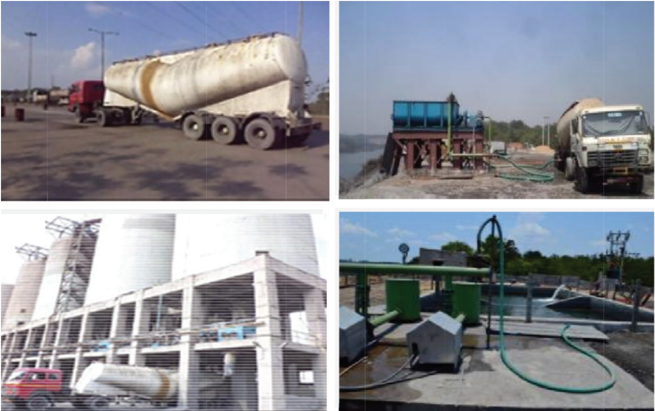
Fig.5 Snapshot of various activities of backfilling operations using conditioned fly ash at mine site
