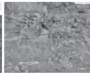
(e) Disintegrated limestone
