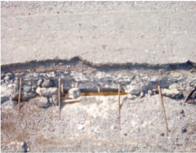
Fig.1 Disease in deck pavement
