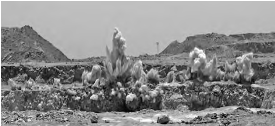
Fig.6 Stemming ejection generated fly rock due to use of without screened drill cuttings
