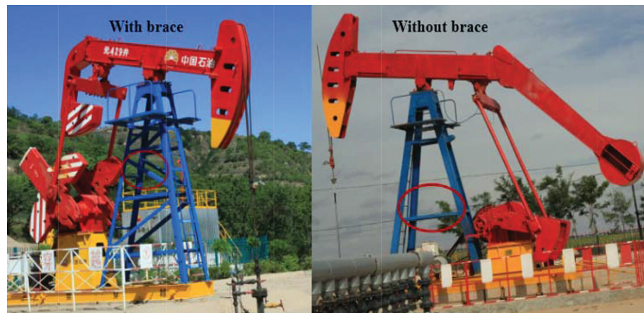
Fig.16: With and without brace of pumping unit bracket
