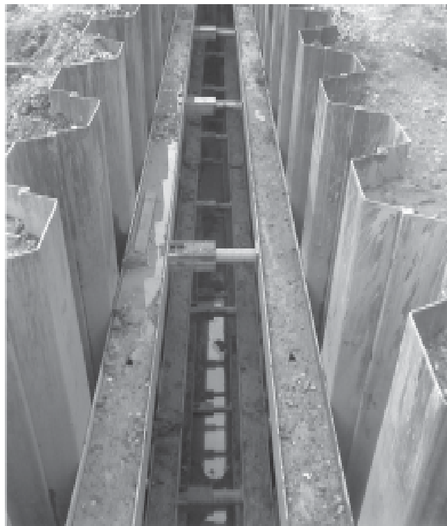
Fig.3 Construction of excavation for a drainage rib supported by sheet pile walls
