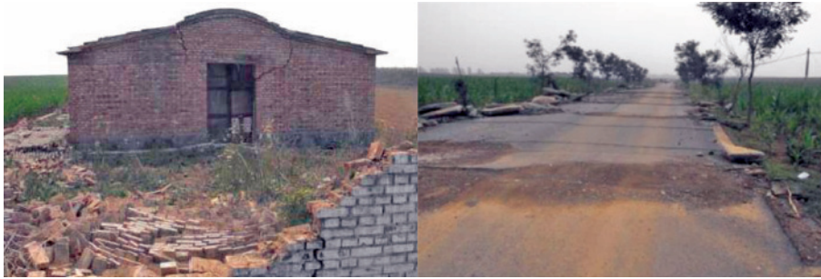
(a) House collapse
