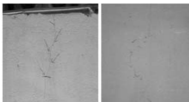
Fig.12 The view of cosmetic cracks developed in the brick-mud-cement house at Kusmunda mine
