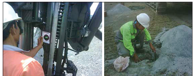
Drilling based on measuring of Auto leveling Pentax Fig.17: Drilling based on measurement of Pentax tool and control depth of drill
