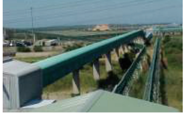
Typical “Totally Enclosed Box Gantry” structure
