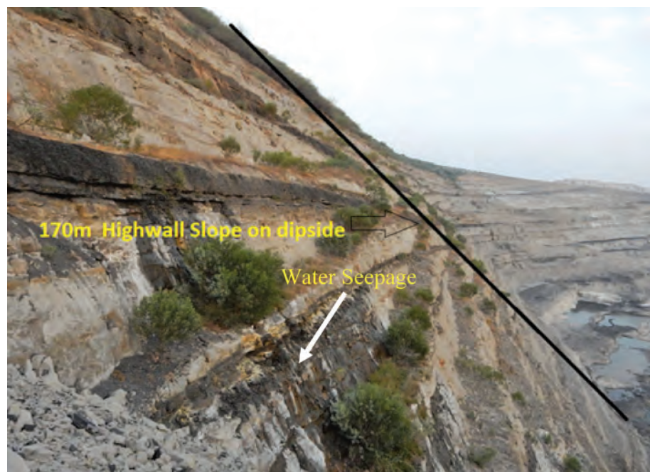
Fig.5(b) Photograph depicting the ultimate slope of 170m highwall of Medipalli OCP
