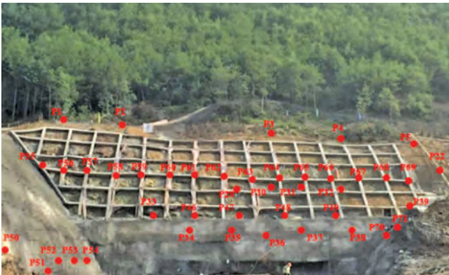
Fig.8 Diagram of surface subsidence measuring points at the entrance of Feilongshan tunnel (part).
