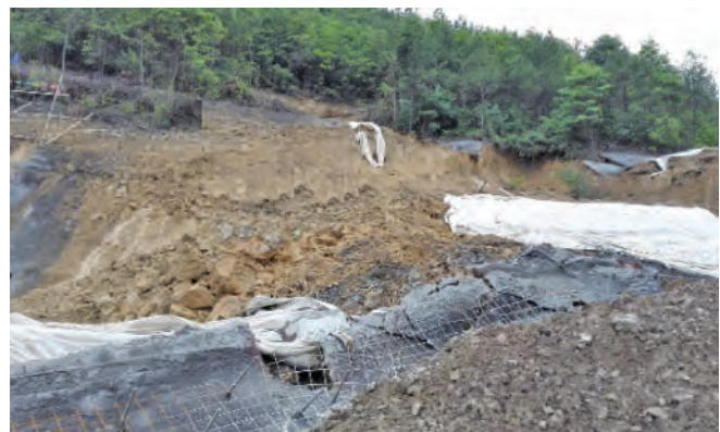
Fig.4 The third-time landslide in the entrance section
