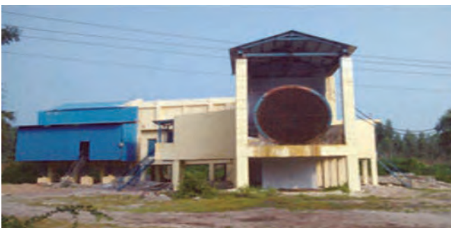
Fig.4 Main mechanical ventilator
