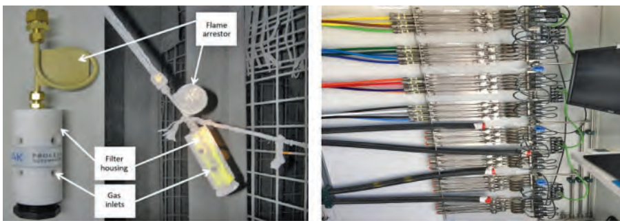
Fig.3 (a) and (b) end of line filter and flame trap at both ends of the tube
