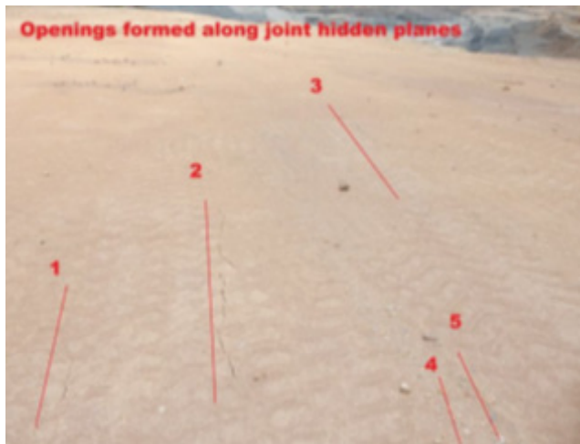
Figure 9. Showing tensional cracks developed on RL870 bench surface.
