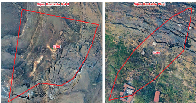
Figure 12: High resolution sample drone image showing cracks present at unstable sites
