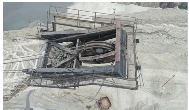
Figure 9. View of the Top pulley of Dragline
