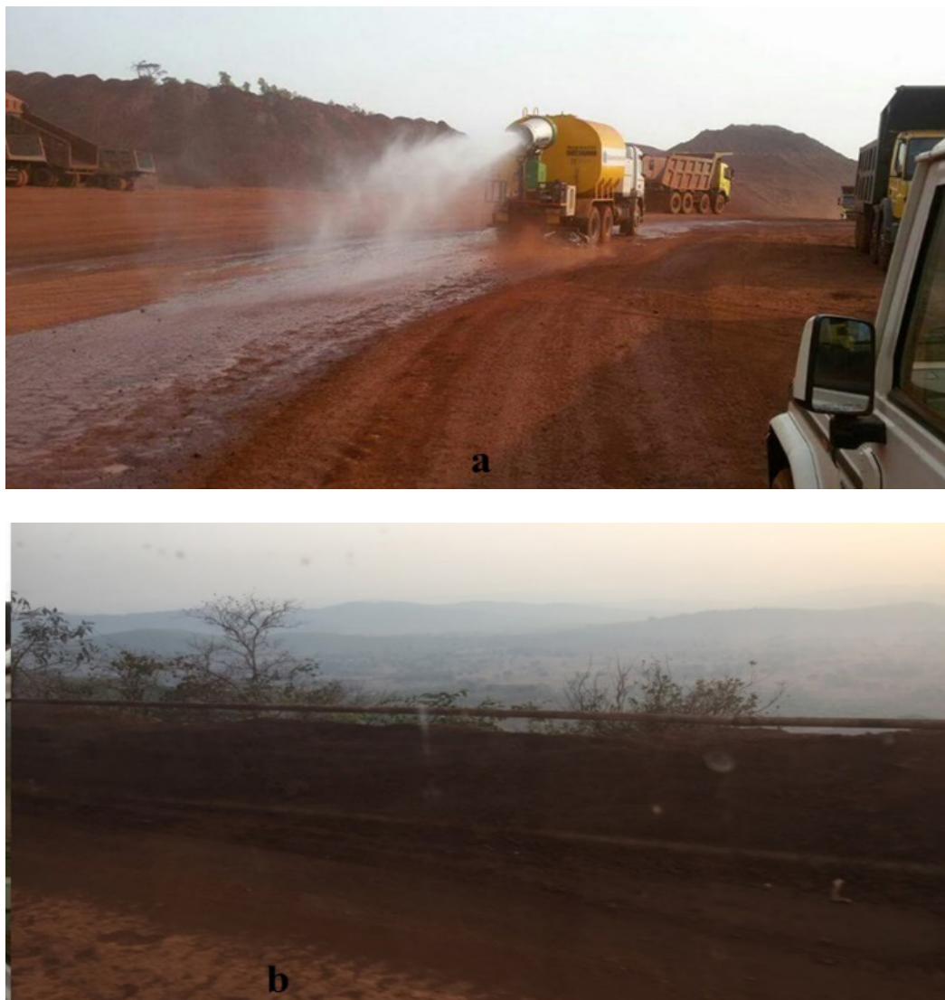
Figure 4. (a) Truck-mounted Mist Cannons. (b) Fixed water sprinklers along the sidelines of haul roads.
